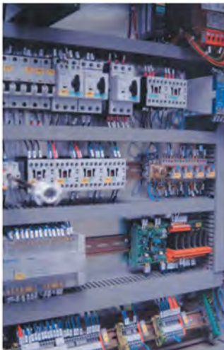
Electrical Box with Numbered Wires This set-up also allows for wiring in options at a later date
